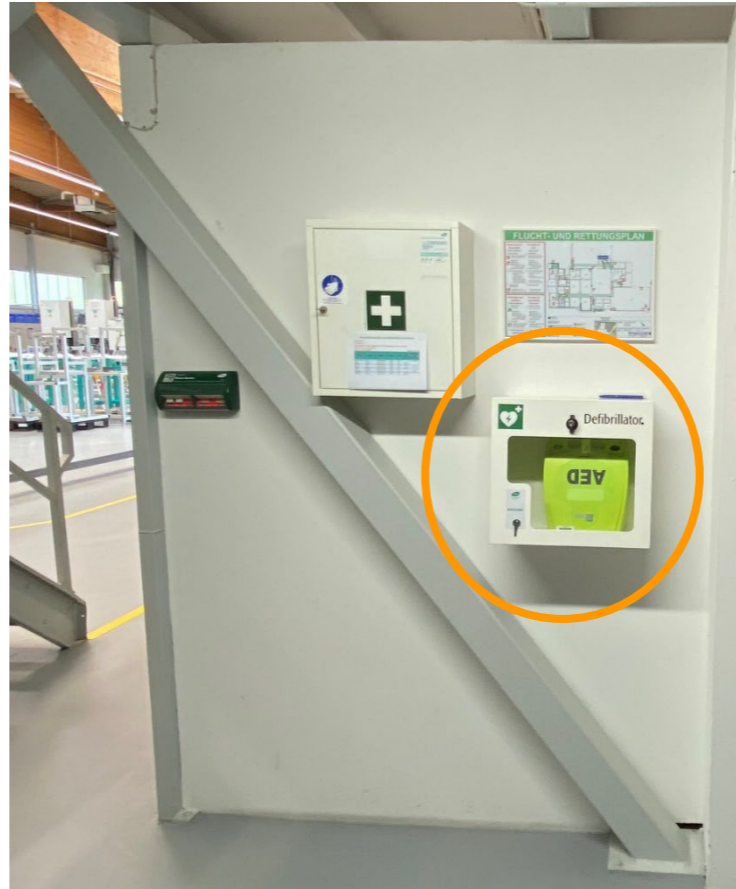
Building 7: at side entrance production (near fire alarm system)
